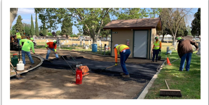
Starting to roll out the hot asphalt, near the recently re-furbished pump house, which was the work of Eagle Scout Joshua Taylor and family.
